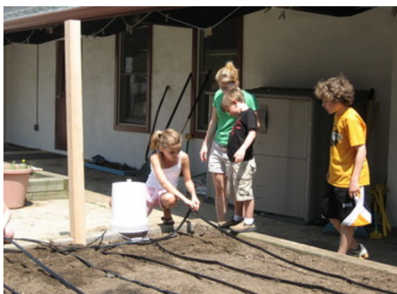
Key School 6 th graders install a drip irrigation system during Earth Week.
